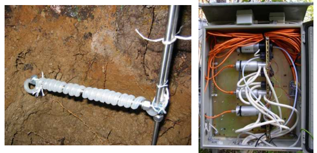
Figure 2. Gas collector installation in the soil (on the left) and the installation box for the GMP343 probes (on the right).
