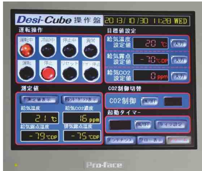
Seibu Giken Desiccant Dehumidifier display (the dew point temperature is shown at the bottom left of the image).
