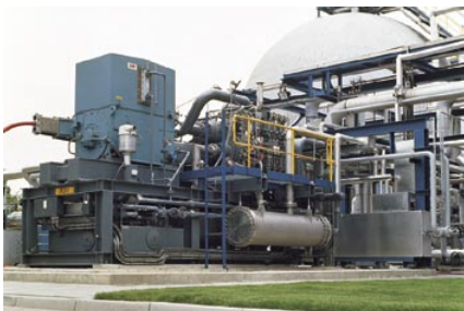
Dew point monitoring of compressed air.
