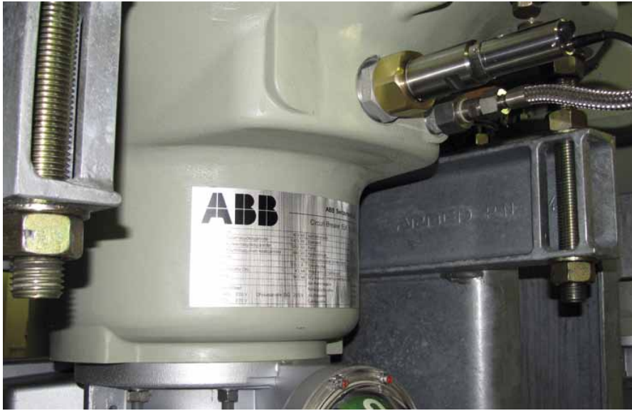
Figure 5. Installation of a dew point-pressure-temperature sensor (DPT145) directly to the main gas tank (25.3– 14.4.2010). The gas volume in the measurement cell is roughly 20 ml.
